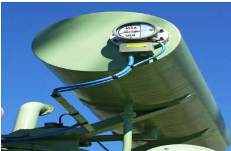
Figure 2 – Conservator oil level indicator
