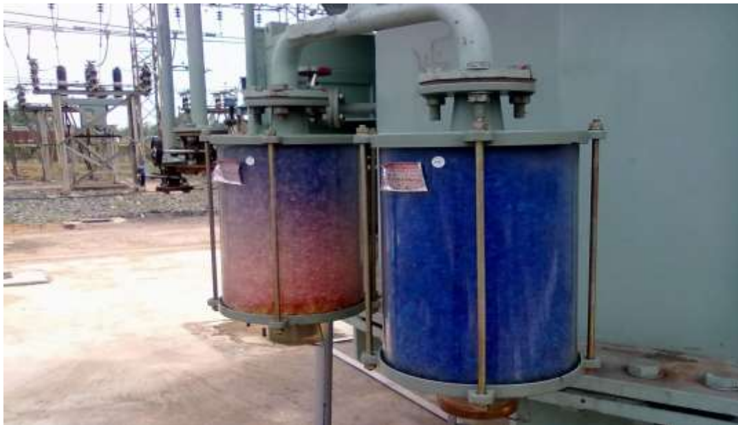
Figure 3 – Transformer silica gel dehydrating breather
